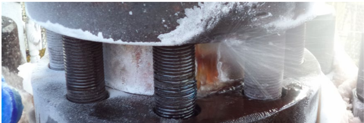
Figure 6: A typical leak of a lens ring flange connection
