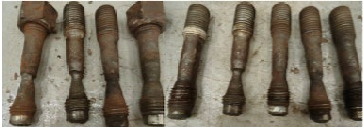
Figure 7: Corroded carbon steel bolts due to a leaking lens ring flange connection
