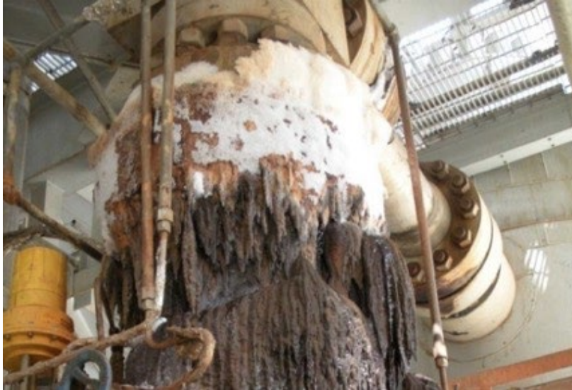
Figure 16: Solids have stopped the leak but created a critical unsafe situation.
