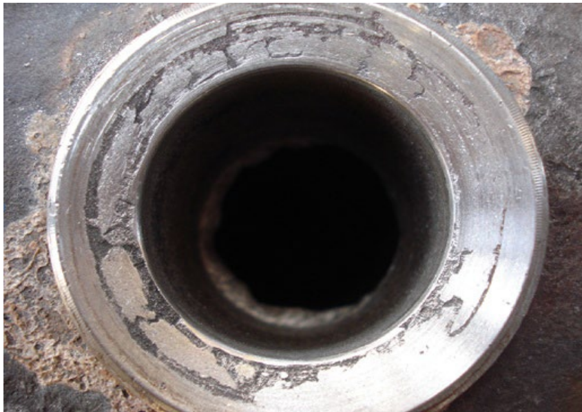
Figure 5: Signs of crevice corrosion of a stainless steel flange face
