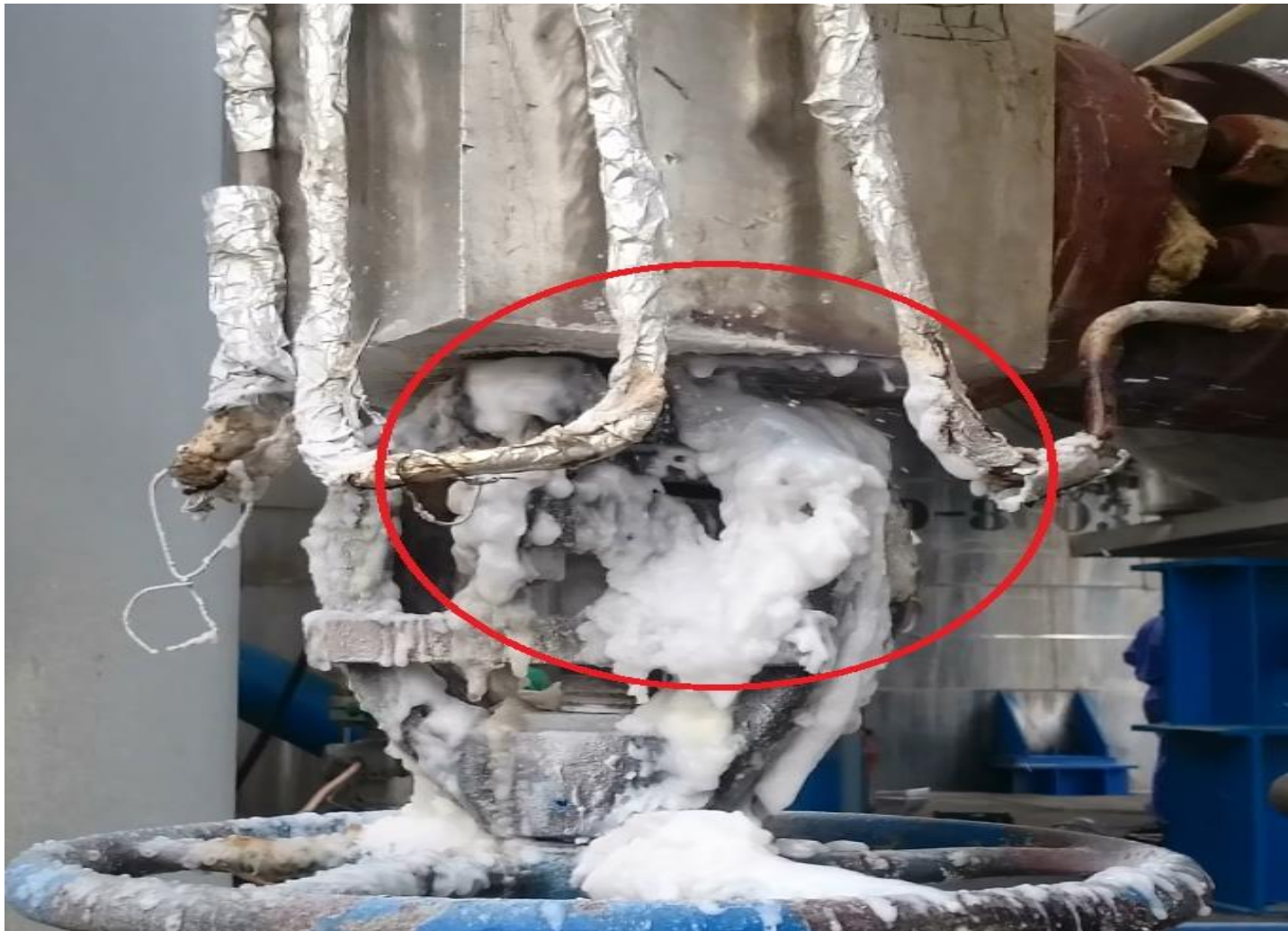
Case 5: A leaking threaded connection of a HP drain valve
