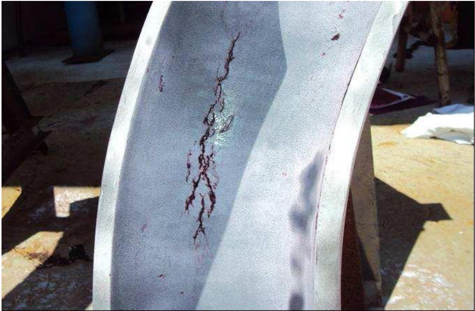
Case 4: Cracks in HP gas line
