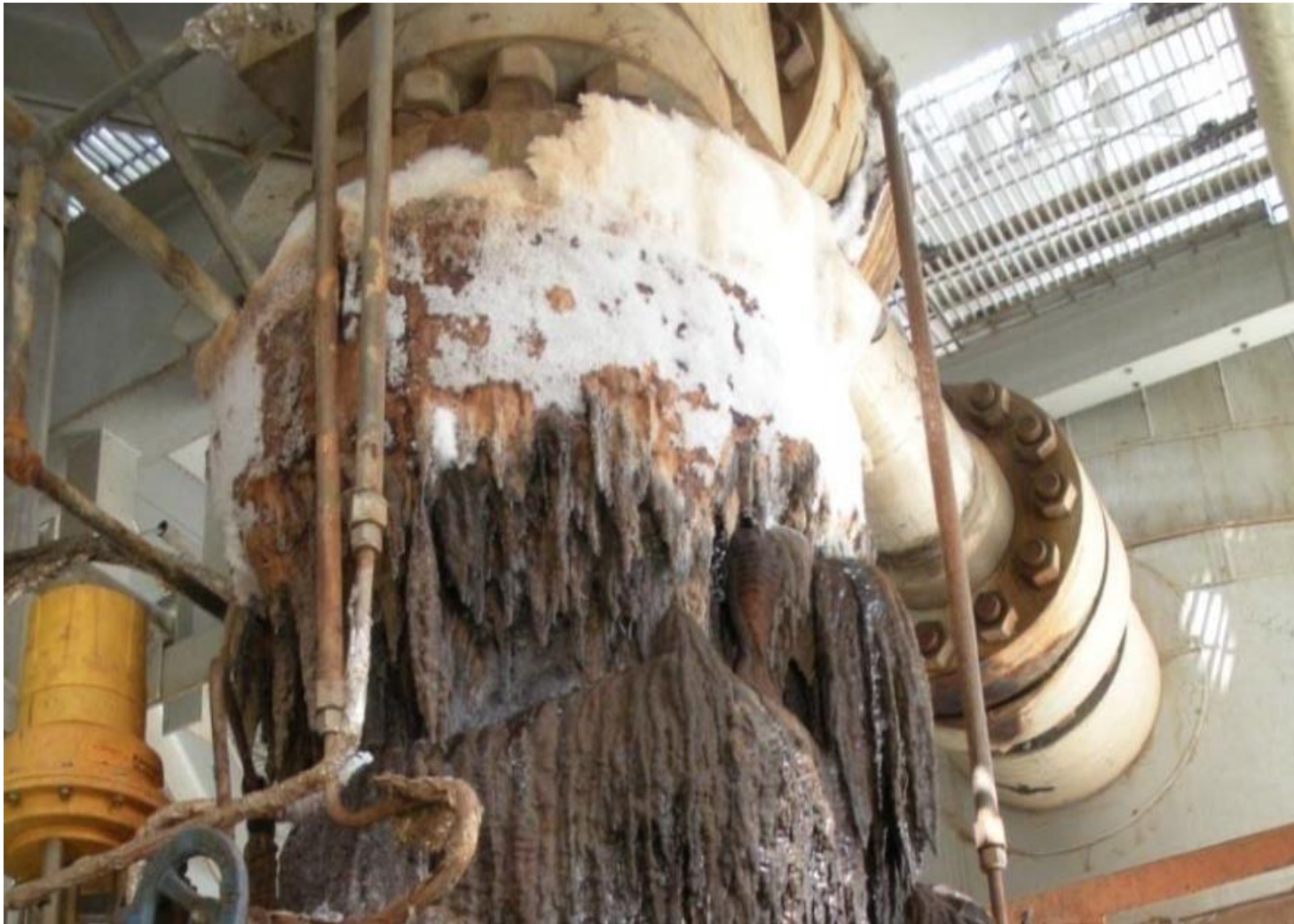
Case 2: A solidified HP flange leak
