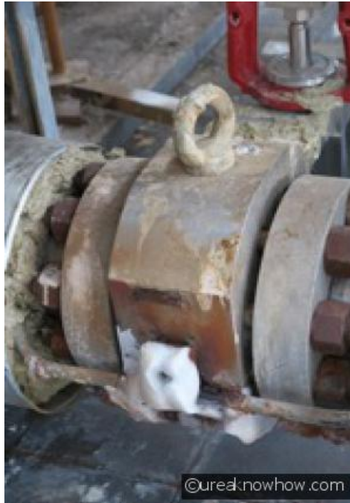
Case 3: A solidified leak along stuffing box of a HP butterfly valve
